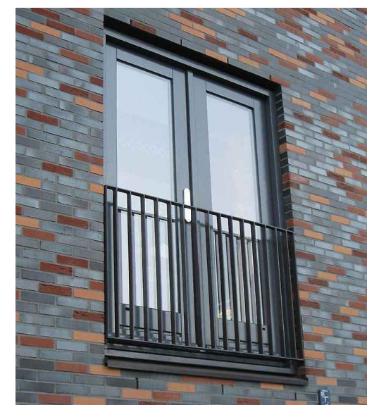
Powder coated metal railing to match balconies, fixed between reveals of opening.
